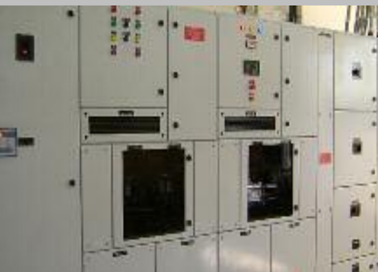
Telecom Switch Room Solutions
